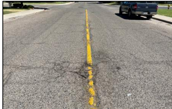
Photo 18: Low severity potholing and high severity transverse and longitudinal cracking transitioning to block cracking.
