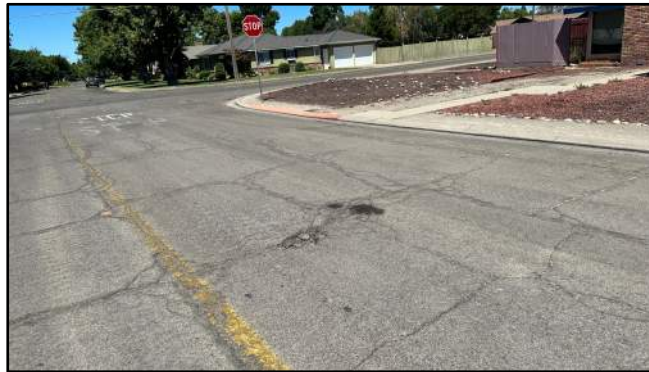
Photo 9: High severity block cracking and low potholing.
