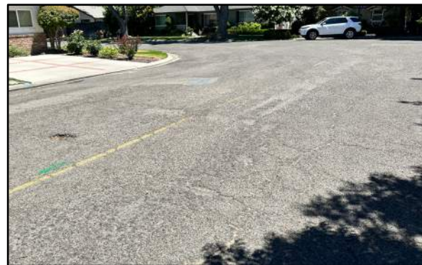
Photo 15: Low severity potholing.
