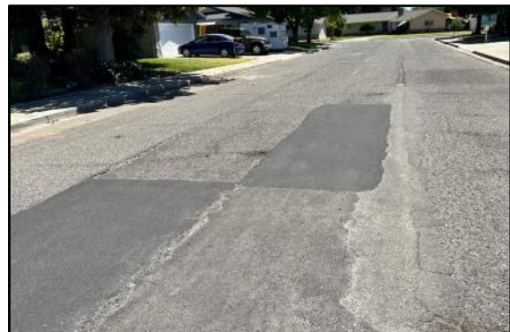
Photo 4: Patches and low severity potholing.
