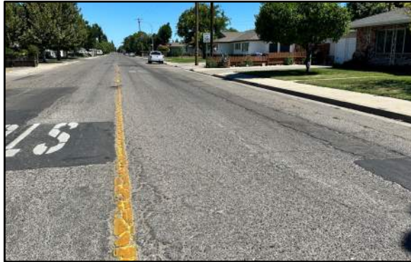
Photo 16: High severity alligator and longitudinal cracking, and patches
