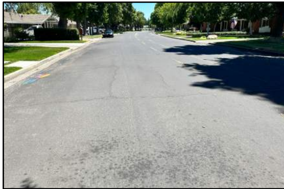
Photo 12: Moderate to high severity block cracking.
