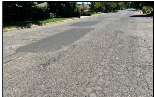
Photo 11: High severity alligator cracking and low severity potholing.
