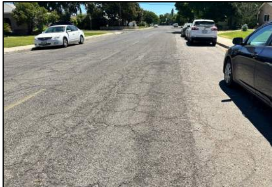
Photo 1: High severity alligator cracking propagating through slurry seal west of Old Vineyard Rd.
