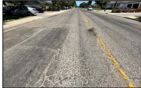
Photo 17: Low severity rutting North of Canal Dr.
