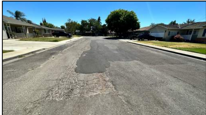
Photo 2: Patches, rutting, and base failure east of Old Vineyard Rd.
