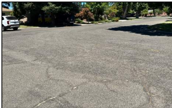
Photo 14: High severity transverse and alligator cracking.
