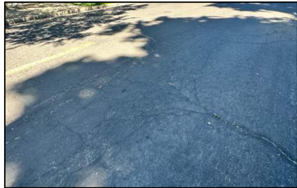
Photo 13: Low severity rutting at potential dig out.
