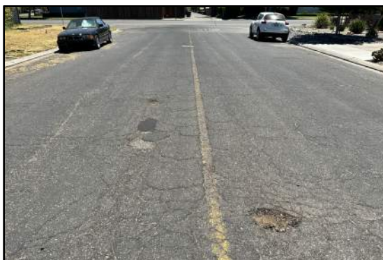
Photo 7: High severity alligator cracking and low severity potholes within existing slurry seal.
