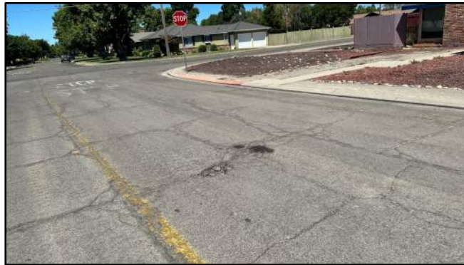
Photo 9: High severity block cracking and low potholing.
