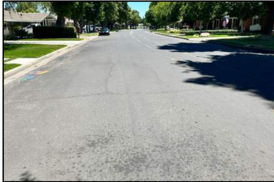
Photo 12: Moderate to high severity block cracking.
