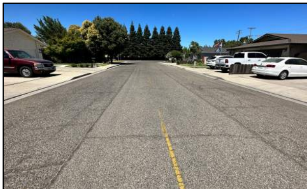
Photo 3: High severity alligator, longitudinal, and transverse cracking.
