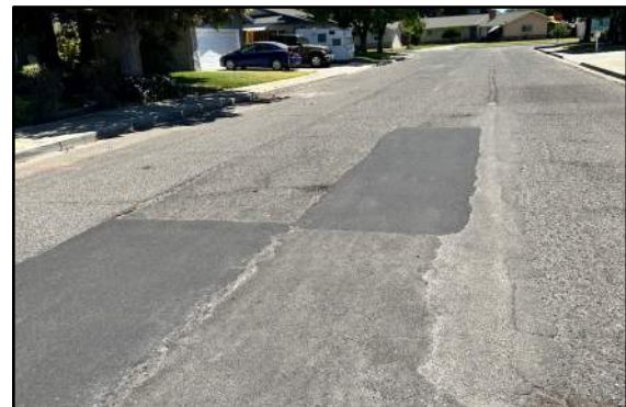
Photo 4: Patches and low severity potholing.
