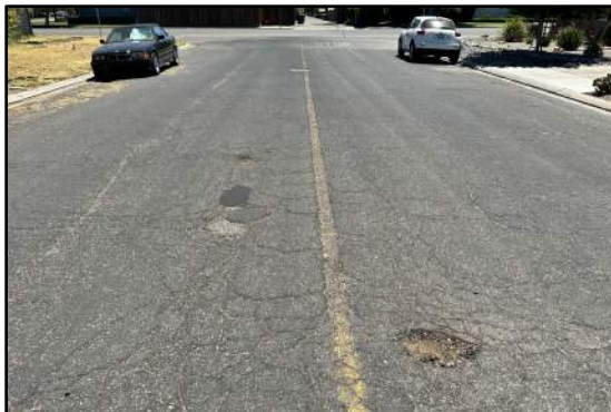
Photo 7: High severity alligator cracking and low severity potholes within existing slurry seal.
