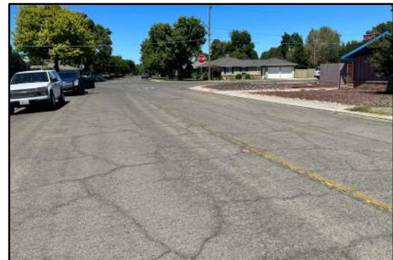
Photo 8: High severity block cracking transitioning to alligator cracking.
