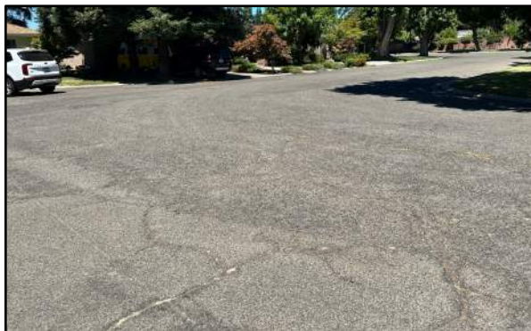
Photo 14: High severity transverse and alligator cracking.
