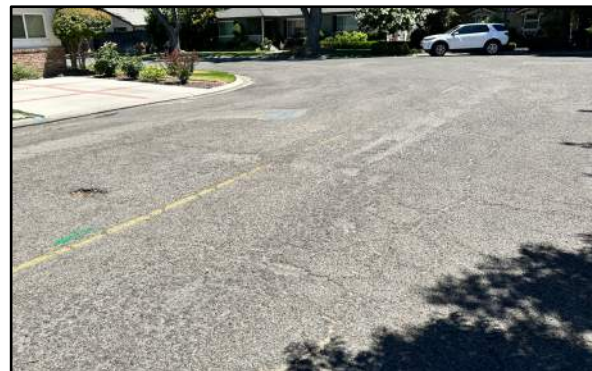
Photo 15: Low severity potholing.
