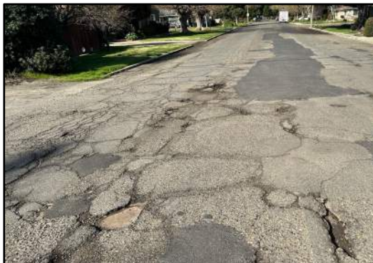
Photo 10: High severity alligator and block cracking, patches, and low severity potholing.
